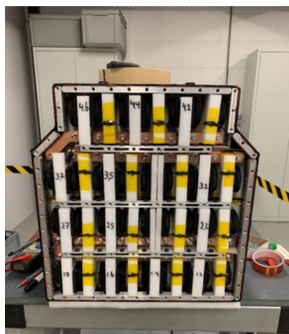
5. A fully connected battery pack with support blocks
